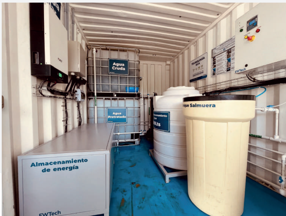
Filtration System and Solar Energy System
